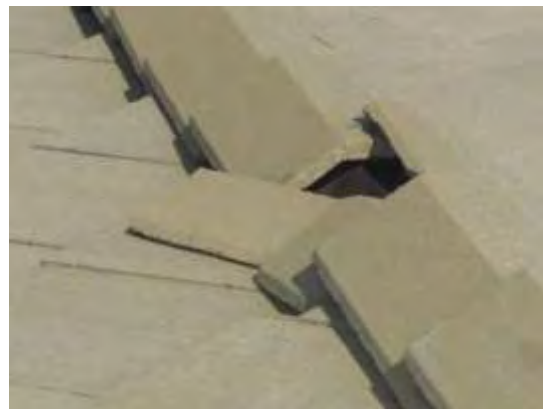
Broken Tile - Typical
