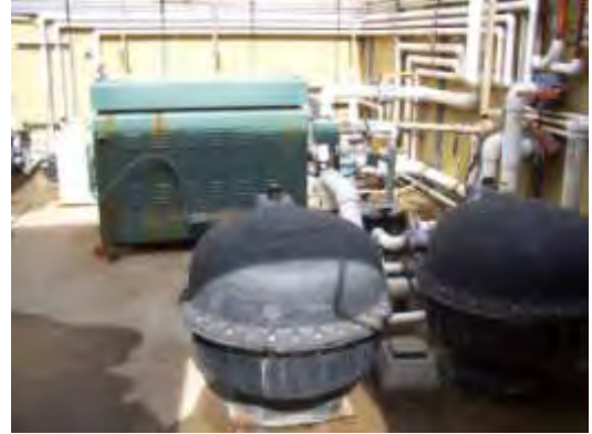
Existing Pool Filtration System
